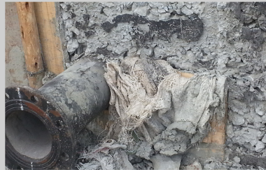
Poor quality casting from an individual contracting approach
